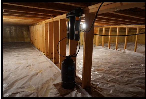
Crawl Space and Water Filtration System
