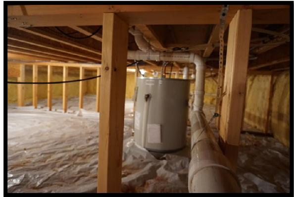
Crawl Space and Water Heater
