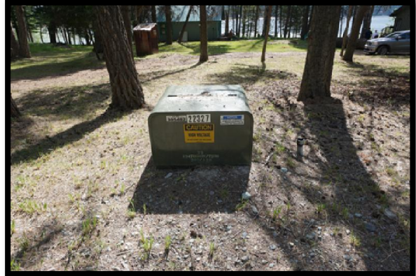
Electrical Utility Box on Property
