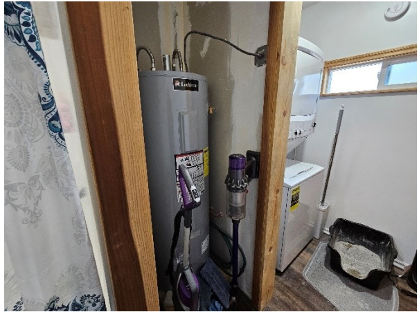
Hot water heater and washer and dryer.
