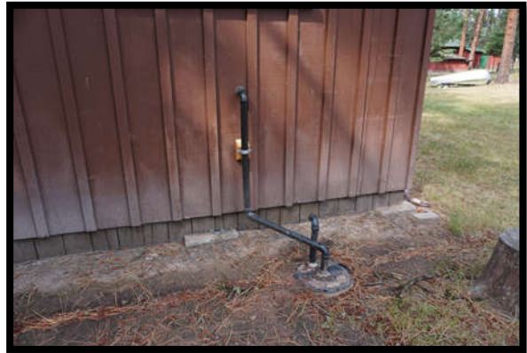
Storage Tank for Kitchen Sink
