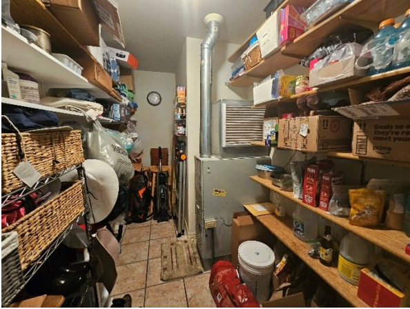
Walk in pantry with furnace.
