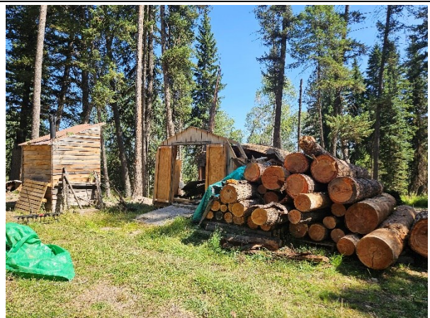
View of a second shed located near the detached garage and outhouse that was damaged in a storm by a fallen tree the prior week.
