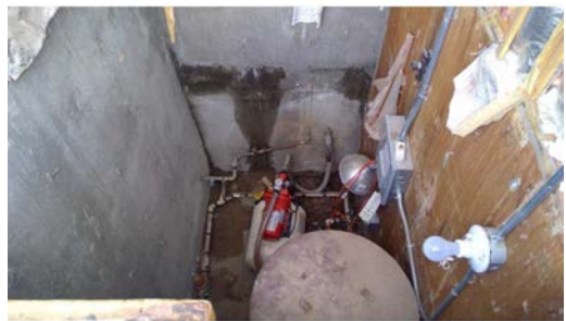
Cistern Pump House
